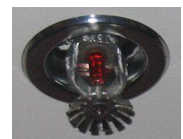
Fire Sprinkler Head (located at ceiling)
