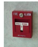
manual pull Fire Alarm System
